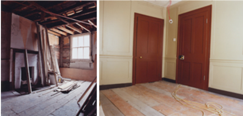
Left: Scholarship Centre - before conservation, April 2005 Right: Scholarship Centre - nearly finished, October 2005
